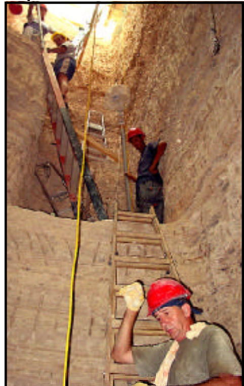
West square pit at 40 foot level as crew continues to descend in search of a paleo-chamber thought to be the anomaly at at the 55 foot level. The pit was dug using two small jack hammers, hand picks, with dirt removed by hand via a bucket chain.
